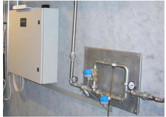
Control Board Automatic CIP cleaning unit.
